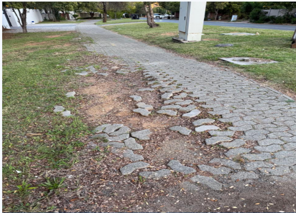
The Randpark Drive walkway — sections in need of repaving
